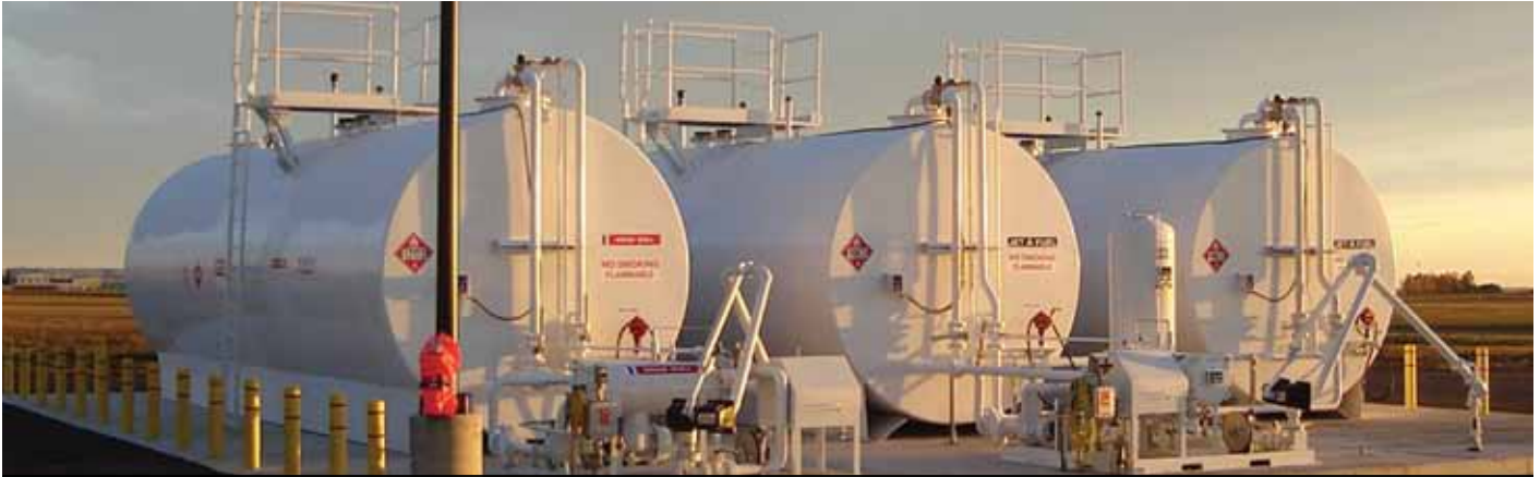
Jet A and Avgas Fueling System
