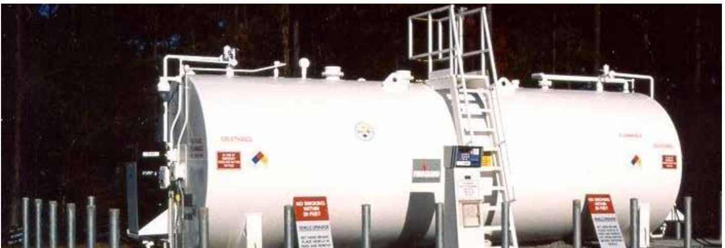
Up to 50,000 Gallon Tank Capacity of E85 or Biodiesel
